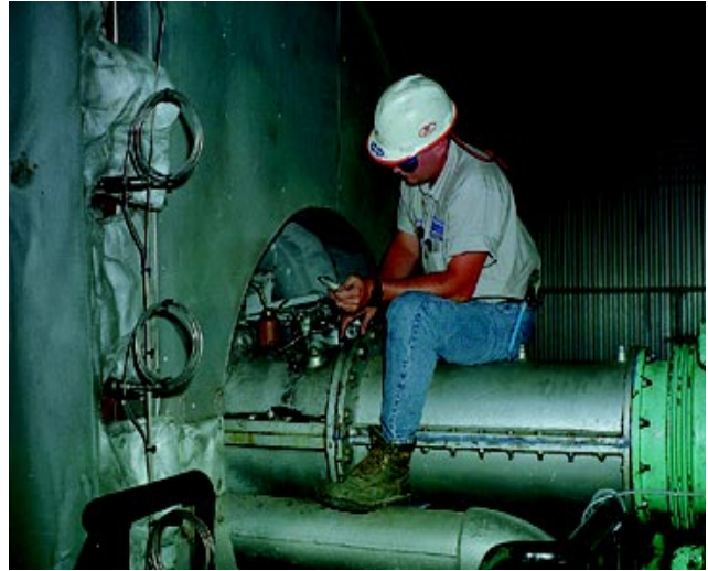
New thermocouple installation (left) and installation of new LP speed sensing probes for gas turbine
