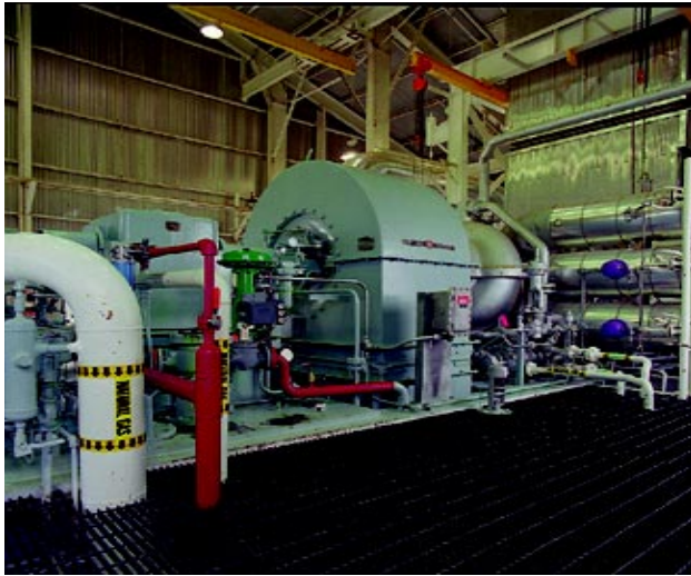
Upgraded fuel valve system, hydraulic system, flame detectors, speed pickups, and thermocouples for gas turbine
