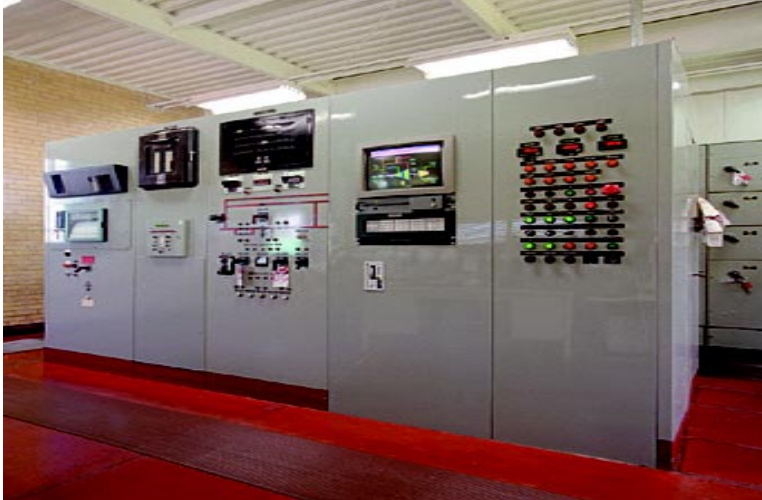
Integrated Control Panels for a GE Frame 3 Turbine Compressor Retrofit Project
