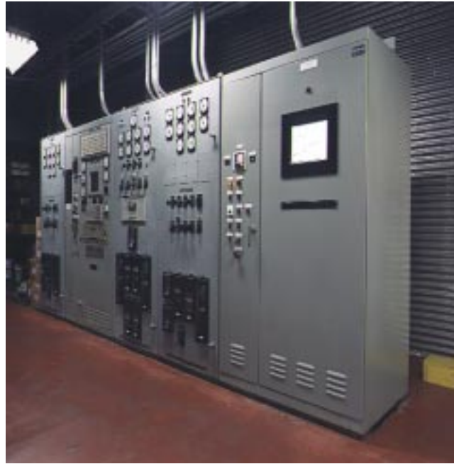
Replacement controls for two Allison 501K generator sets in emergency backup power service
