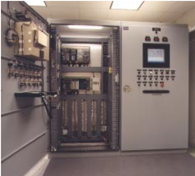
Replacement controls for two Ruston TB4000 gas turbine driven pumps for crude oil pipeline service
