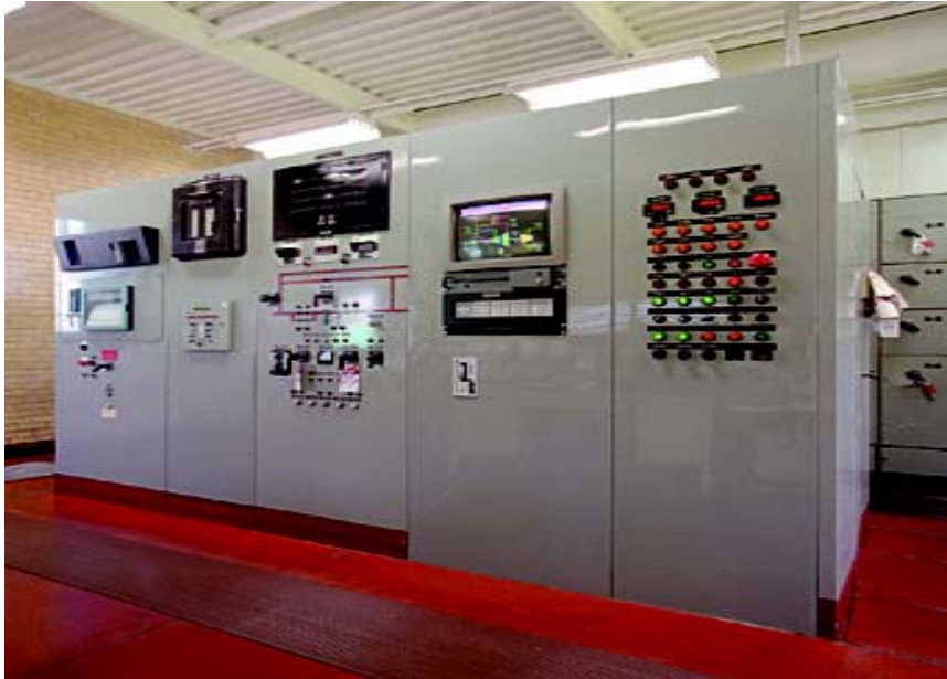
Integrated Control Panels for a GE Frame 3 Turbine Compressor Retrofit Project
